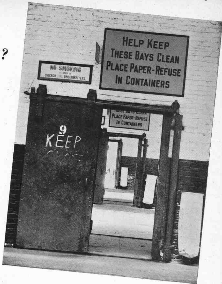
It won't happen here—no litter of waste-paper to feed a fire in these bays. These signs and receptacles installed experimentally at Kedzie met with immediate cooperation from the trainmen, with the result that similar set-ups are being made at the other stations. Each bay has a waste bag by each entrance door. Easily emptied, the containers help solve a difficult cleaning problem.
