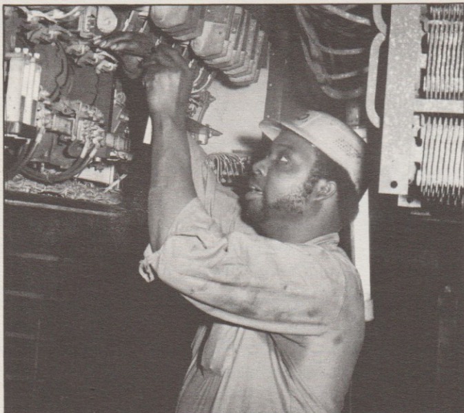
Car repairer Robert Calhoun of 98th Street Terminal makes adjustments to electrical components. Safety equipment, such as the bump hat which Calhoun wears, is second nature to repairmen and other maintenance personnel.
