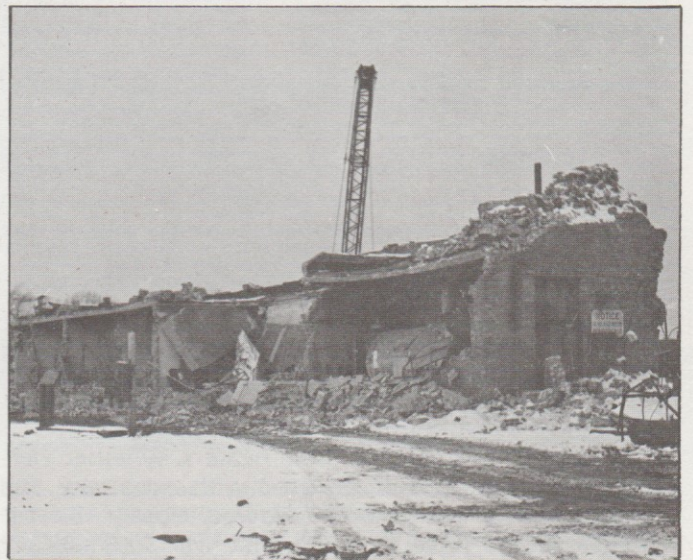
A wrecking ball, hoisted from a crane in the background, makes short work of the demolition project at North Avenue as the building crumbles under the weight of the ball.
